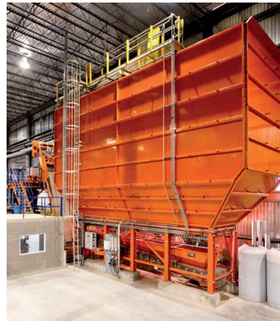
This four-compartment aggregate storage system is located inside the Lecuyer pipe plant to protect aggregates from the harsh Canadian winter. Aggregates are dumped by truck into an outside ground-level hopper and conveyed inside to a four-position transfer belt that automatically loads the appropriate bin with sand or stone. Two cement silos are located outside.
