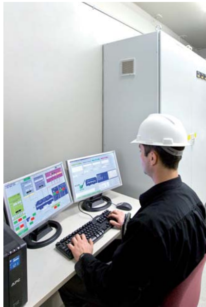
The ACT PCS Programmable Control System uses a graphical point and click user interface and keyboard to control the ACT MobilMat batching plant. The PC based system uses a programmable logic controller (PLCs) to control every part of the batching/mixing plant. Once set, the plant runs unattended with extreme precision.
